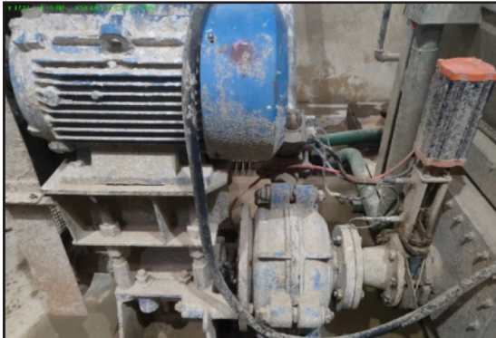
Before – Fluid cement pump with leakage.
